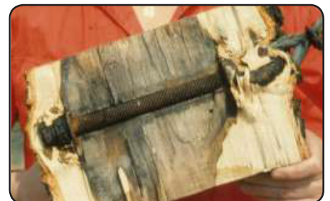
Dark area shows decay commonly associated with bolts used to attach steel cables.
