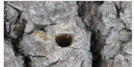
D-shaped borer exit hole.
